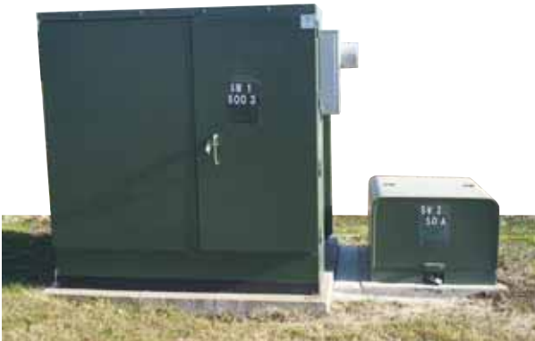
3-Ø Padmount Transformer
