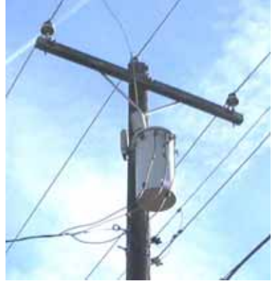
1-Ø Overhead Transformer
